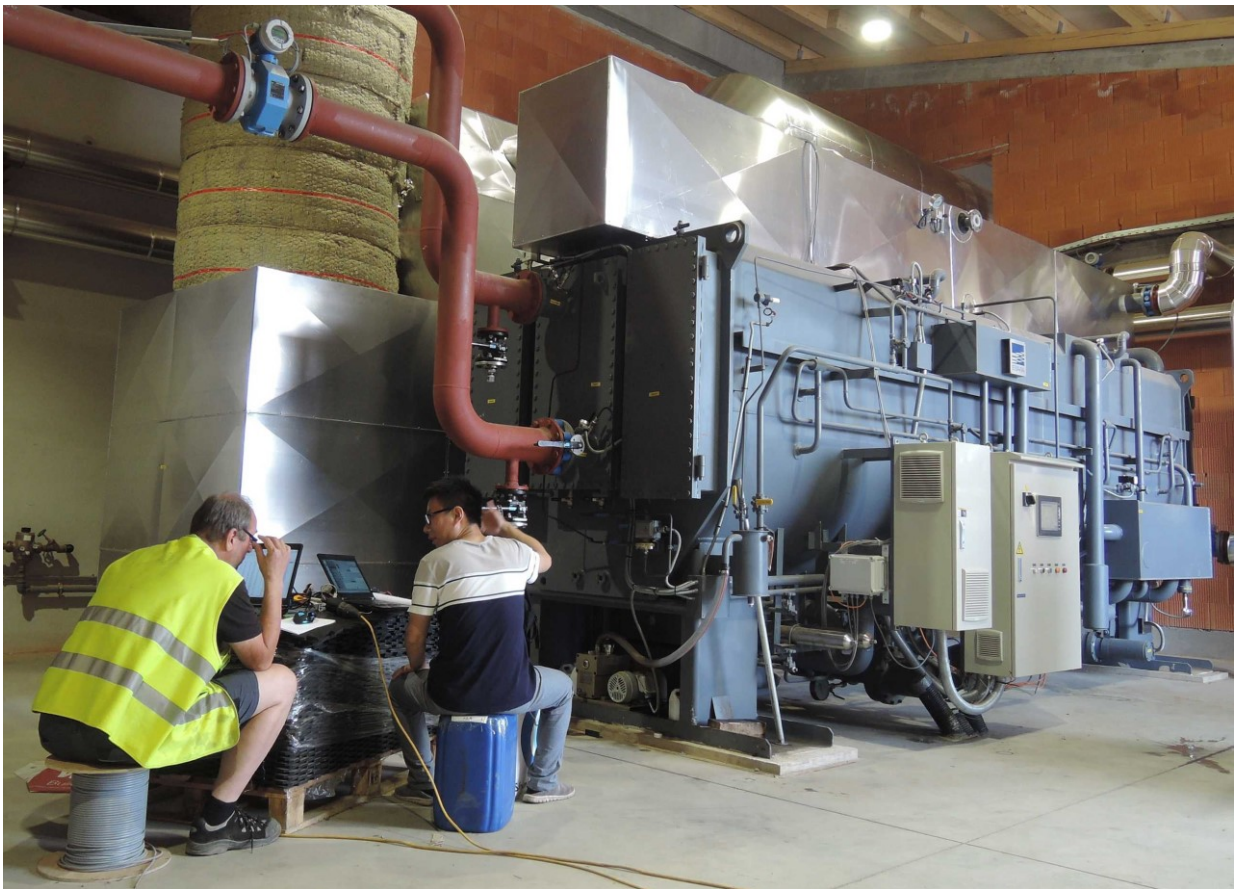
Absorption Heat Pump, © StepsAhead
